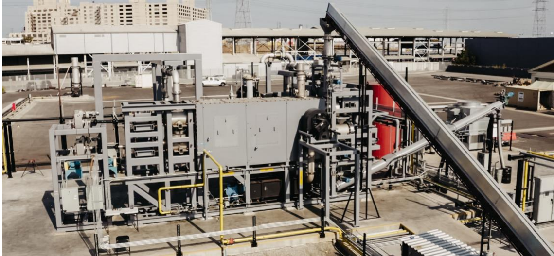
Kore commercial scale facility in downtown Los Angeles converts 1 ton/hour of feedstock into carbon negative Biogas, Hydrogen, and RNG and Biocarbon.
